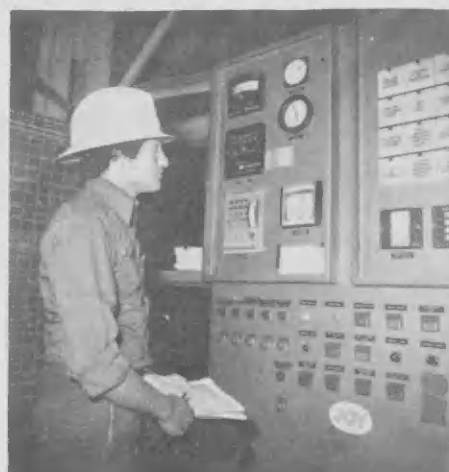
Mario here studies the panel of Joy Compressor at No. 2 Powerhouse.
